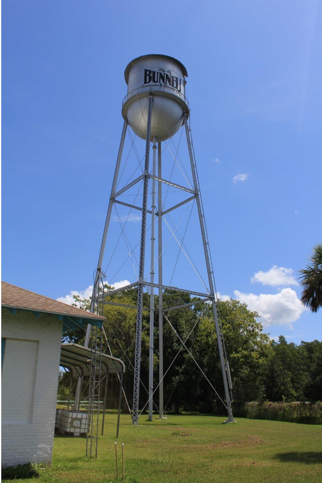
Figure 9 – NW Side – Full View of the Water Tower – (photograph by author – August 2018).
